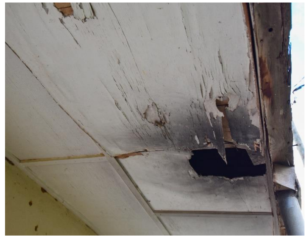
Leaking ceiling at bitereko office
