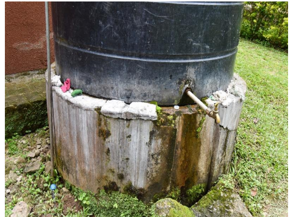
Tank Base at Kalinzu sector to be renovated
