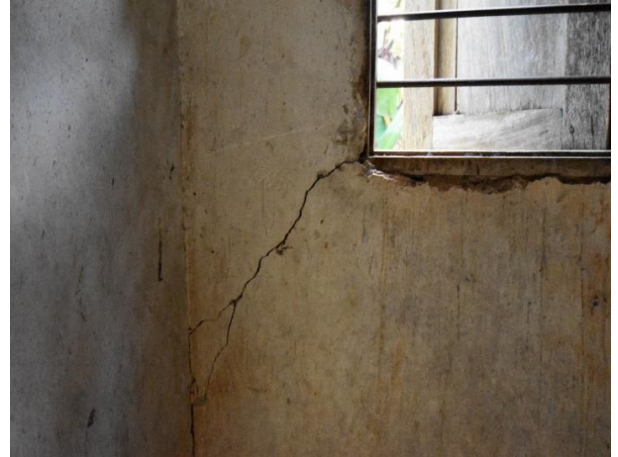
Structural cracks discovered at Bitereko
